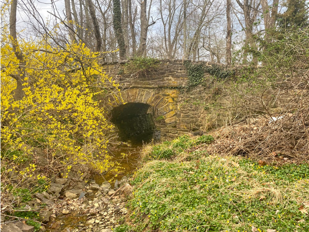
Photo 4: Federal Twist Road stone-arch bridge, Overall view of the west (upstream) side, view facing east.
