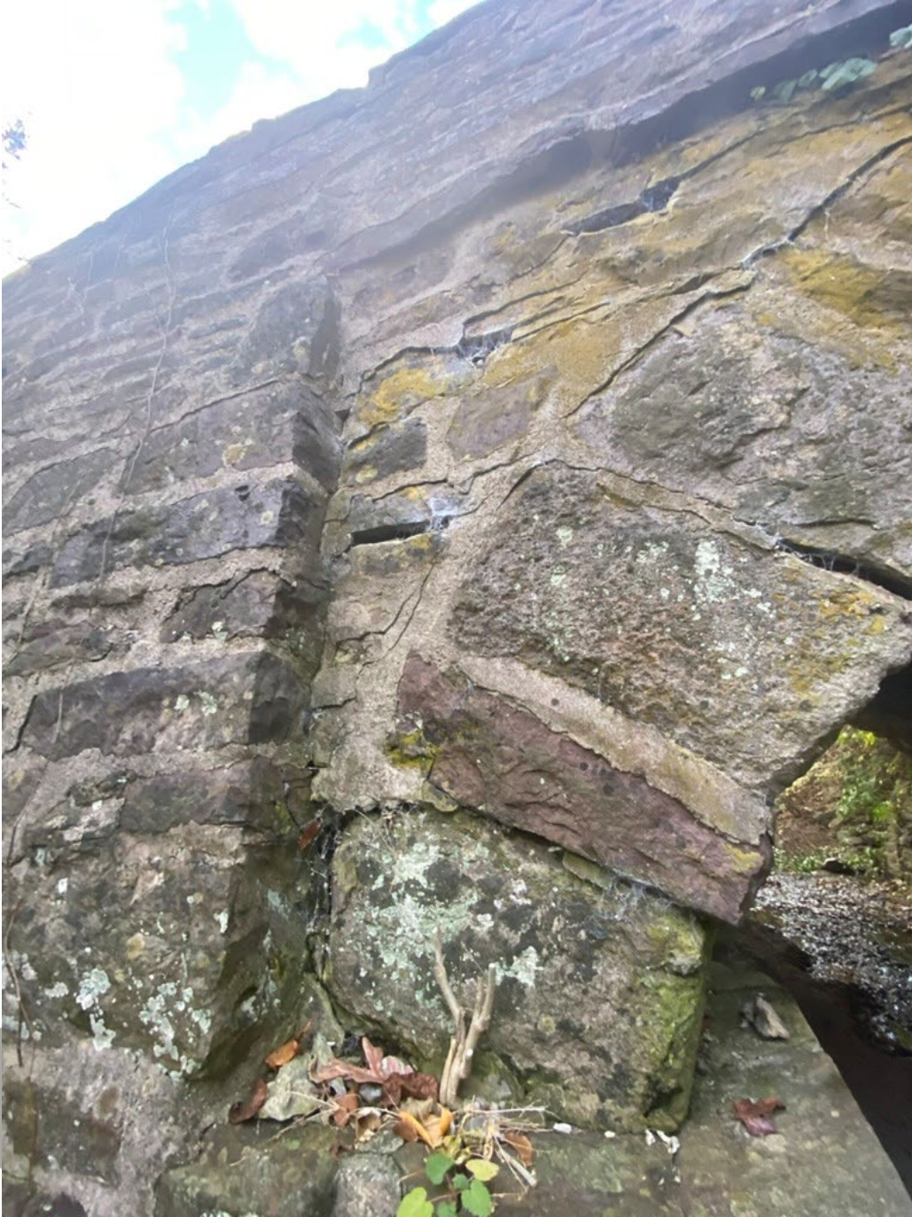
Photo 7: Federal Twist Road stone-arch bridge, east (downstream) side, view facing west showing the quoined corners of the inset panel.
