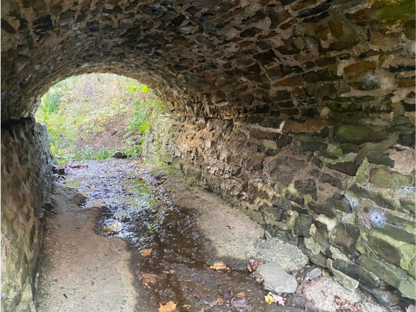
Photo 8: Federal Twist Road stone-arch bridge, view facing west showing the arch barrel and the battered stone bases.
